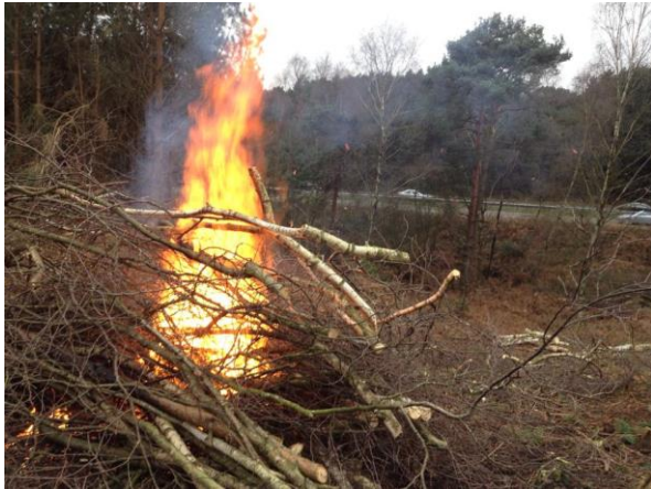
Heathland restoration in Dorset, as mitigation for A338 road widening (Photo: Noel Bergin).
