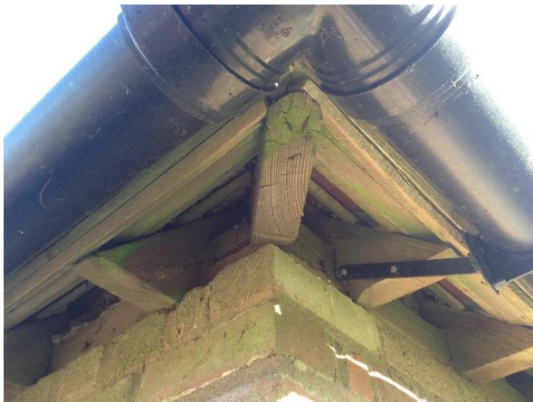
Open eaves on a cottage roof in Surrey, allowing potential access to bats (Photo: Alice Quinney).
